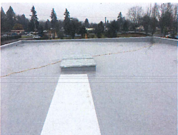
Roof progress Welded and fully adhered roof installed with walk pad to mechanical equipment
