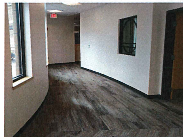
Interior progress Looking toward lobby-note window which remained throughout the project. The contractor actually removed the window and re-framed it to match the other new windows at no cost to the county
