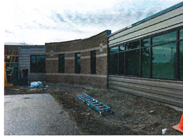
Roof progress Cap flashing at parapet wall is being installed and windows are in
