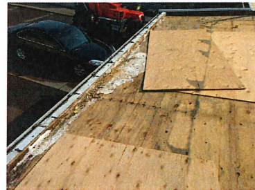
Phase 2 Rotted insulation curb block and plywood decking
