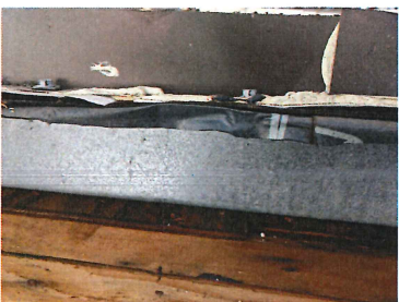
Phase 1 Wet plywood at the top of the wall All along the top of wall above low slope roof had signs of water infiltration which had a path under the roof and vapor barrier
