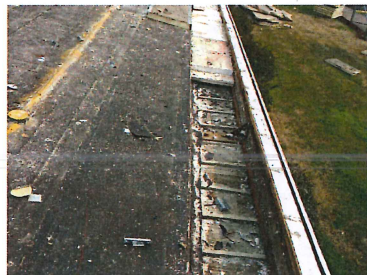
Phase 2 Demo of old roof exposing soffit being filled with insulating foam and no structural wood
