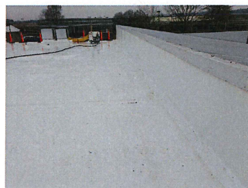
Phase 1 Final low slope roof forming continuous seal to the top of the wall
