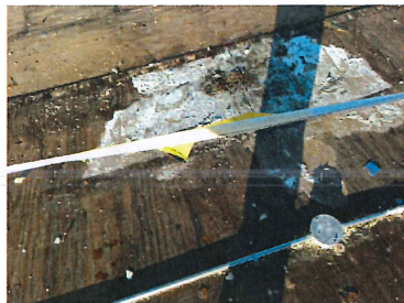
Phase 2 Rotted plywood found during demo
