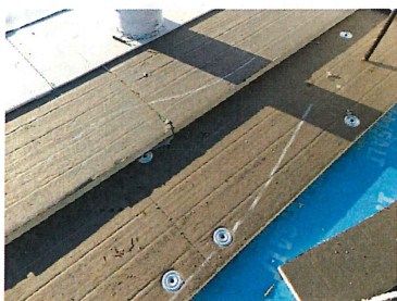
Phase 1 Display of roof system layers-Vapor barrier (blue), first layer of 2" insulation mechanically fastened, second layer of 2" insulation adhered with adhesive, cover board and roof membrane fully adhered
