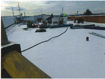
Phase 1 Bulk of low slope roof completed and demo of metal siding
