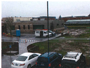
Exterior progress The finished exterior-view from the 2 nd floor of existing administration building
