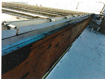
Phase 1 Wet plywood and water pooling in the flashing
