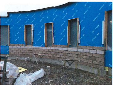
Exterior progress CMU and vapor barrier in progress-note roofing material hanging over parapet wall
