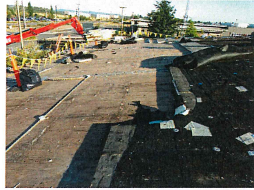
Phase 2 Demo of old roof system. No structural plywood, only 30 pound roofing felt, no self sealing vapor barrier over electrical conduits, no cover board and thinner insulation is what was found
