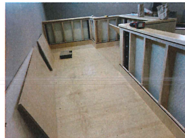
Interior progress Note the ballistic armor inside the walls of Judge's bench and removable panels for electrical access
