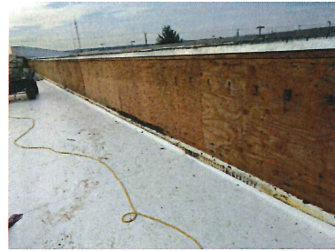
Phase 1 Metal siding removed so roof material can be adhered up and over the top of wall
