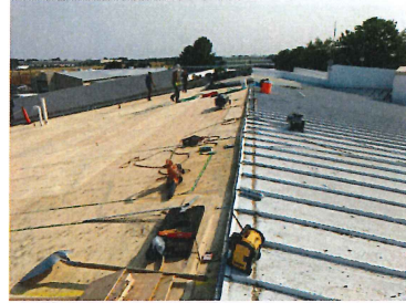
Phase 2 Roof with new structural plywood added-preparing to install self sealing vapor barrier
