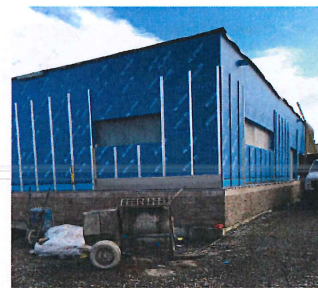
Exterior progress Furring strips for metal siding to attach to leaving a rain plane for any condensation to flow out
