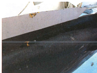
Phase 1 Moisture pooling on vapor barrier at top of wall
