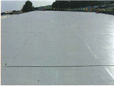
Phase 2 View looking toward jail on East slope of fully adhered and welded membrane. Note ridges of cover boards
