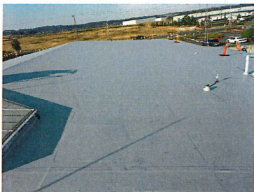
Phase 2 View looking toward Aumsville Hwy on West slope of fully adhered and welded membrane. Note ridges of cover boards
