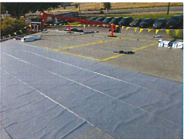
Phase 2 New self sealing vapor barrier installed with yellow paint identifying where electrical conduits lay
