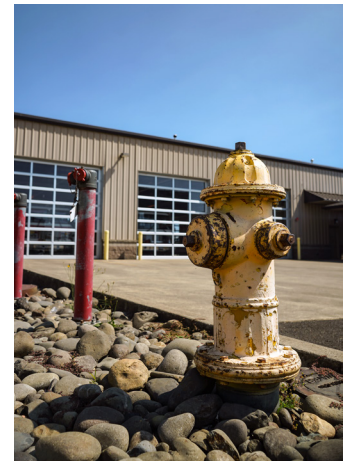
These hydrants outside the Brooks fire station are part of the water infrastructure being upgraded in the community.
