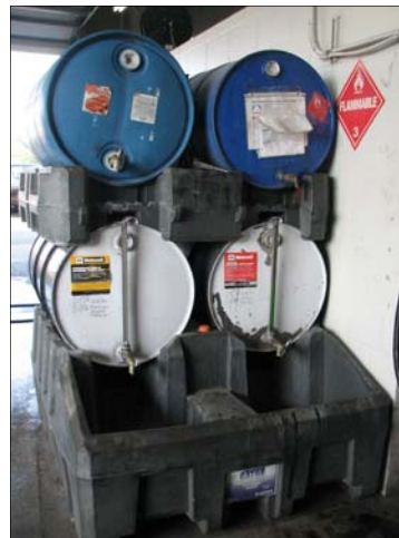
55 gallon drums of coolants, degreasers and cleaners are purchased instead of small containers. They sit in a specially designed rack to catch any leaks.
