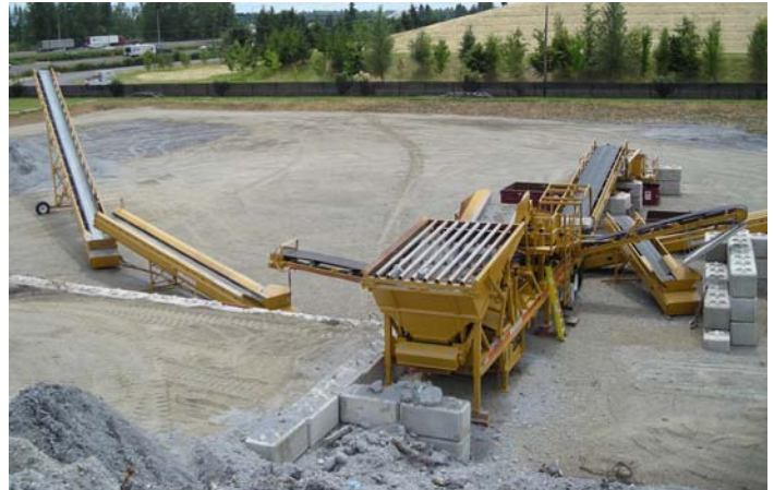
The screening plant
